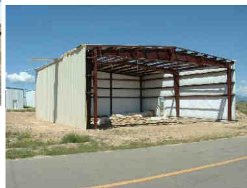
Most of the structural steel was up by late July. Photos by Don Gillmore
