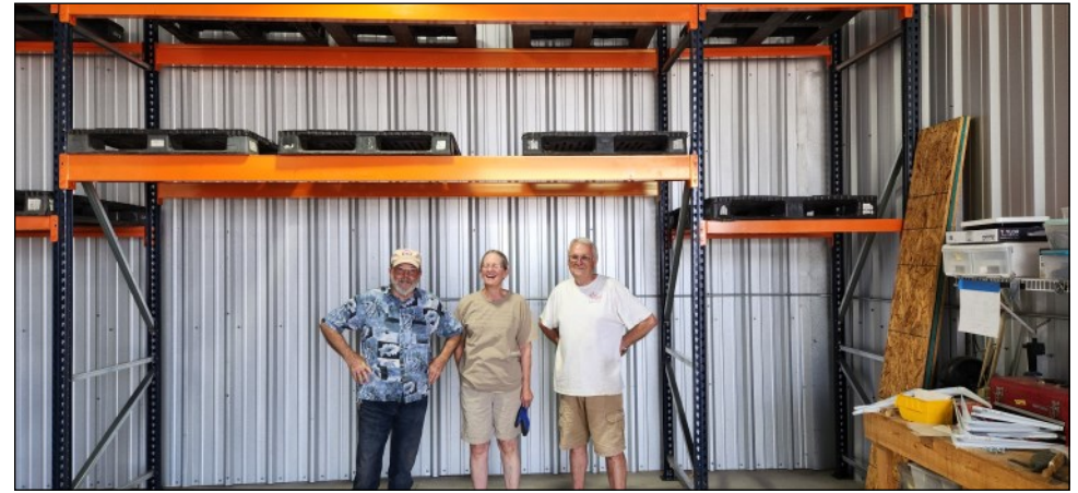
Part of the Upgrade Crew with their handiwork—installing the robust shelves in the back of the RAF. Stephen and Meg Fleming, and Lee Otto.
